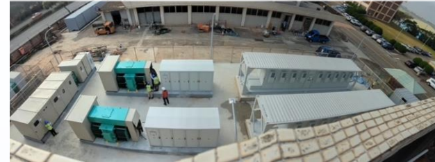
Energy Storage System 2nd and 3rd sites
